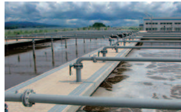
General Water Treatment
