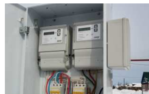
Automatic meter reading
